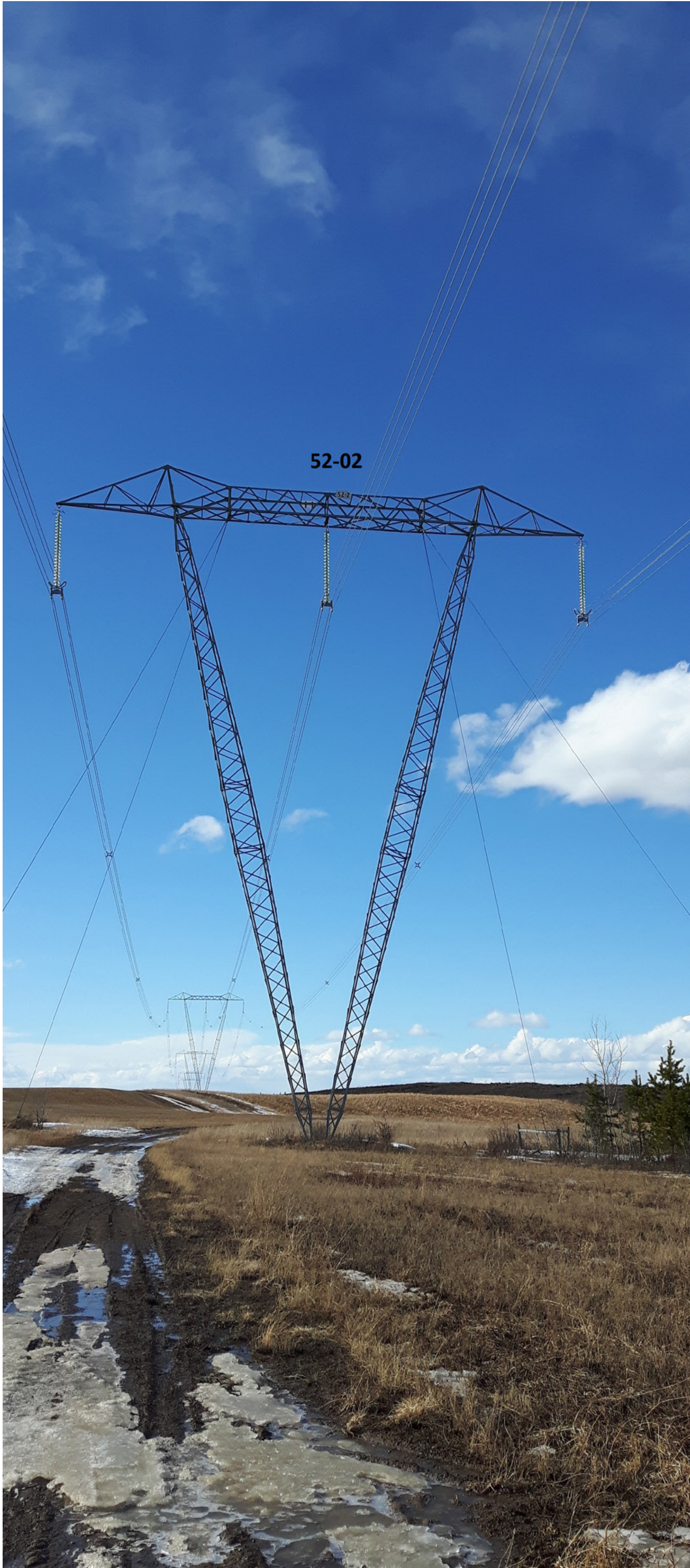
Existing 500kV transmission line
