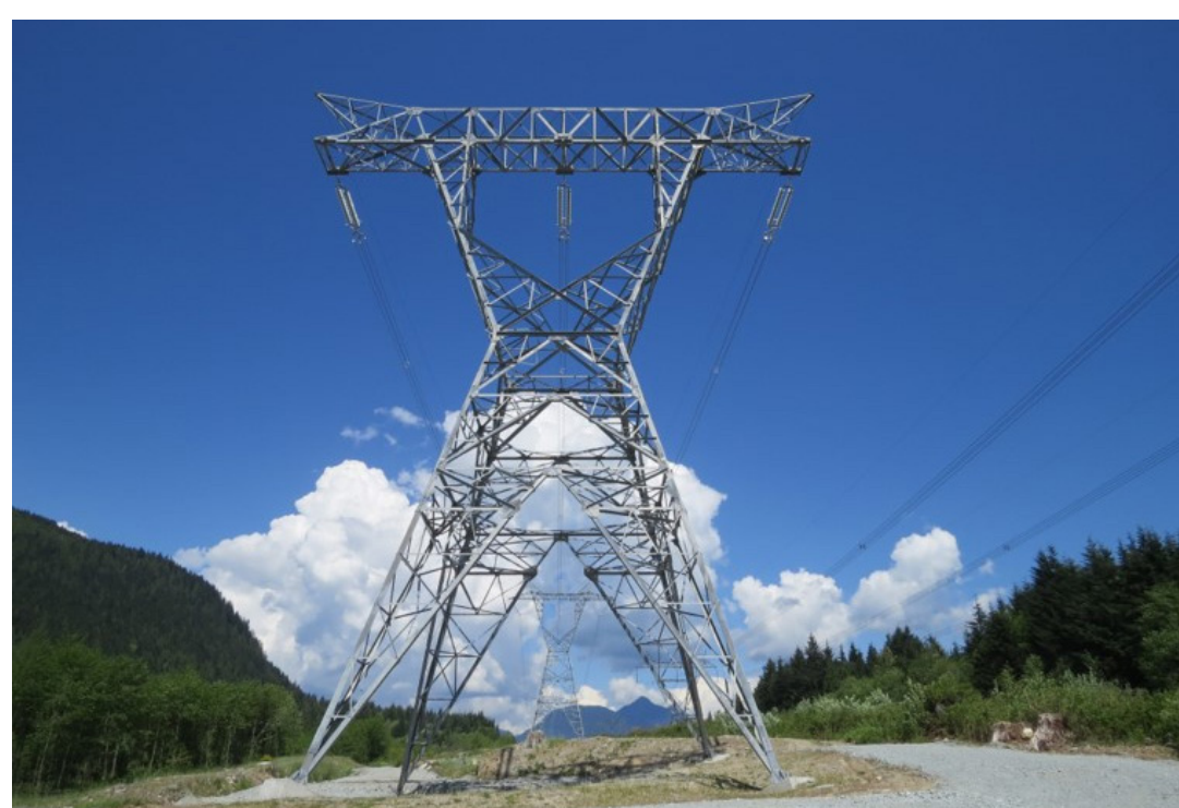
Self Support Lattice Dead-End (most towers in steep terrain)
