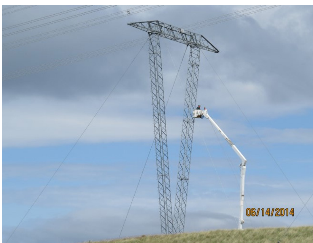
Lattice Guyed Flat Tangent (most towers from Glenannan to Telkwa, and in flatter areas from Telkwa to Skeena)
