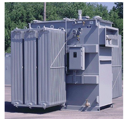
Example of a medium voltage transformer
