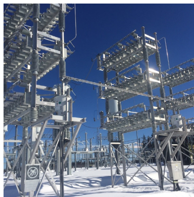
Example of a shunt capacitor bank
