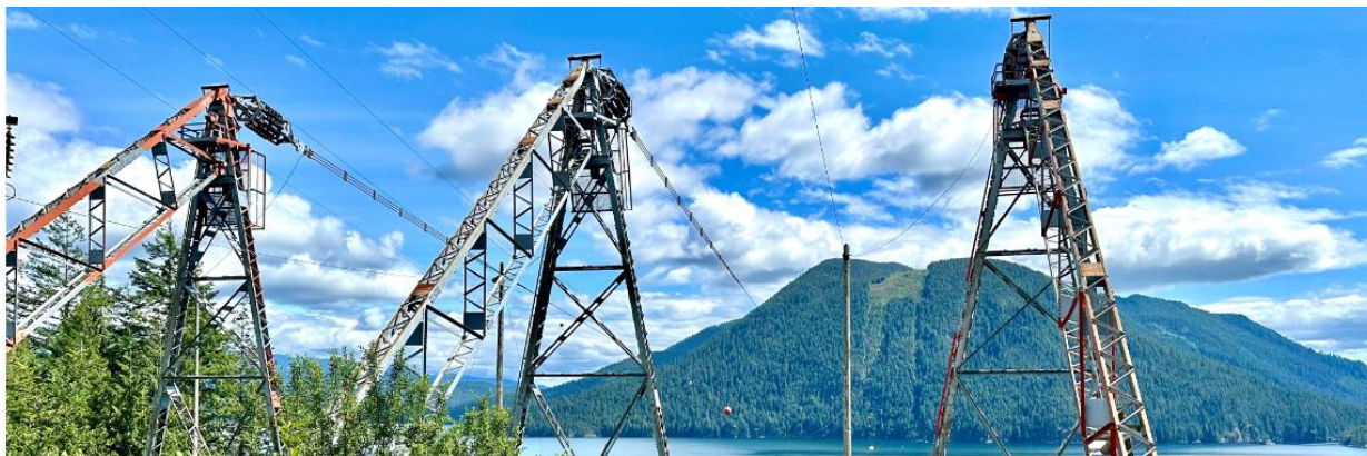
Jervis Inlet North – 138 kV line.
