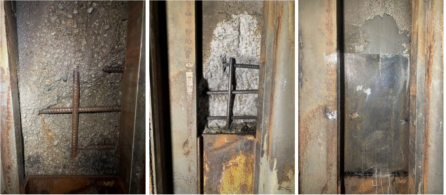
Figure 6 Terzaghi Low Level Outlet Gate #1 guide repairs. Left: Concrete deterioration with exposed reinforcement in the guide slot. Middle: Completed removal of delaminated concrete, surface preparation, and rust cleaning from the reinforcement. Right: Welded steel plate installed in the slot, with the concrete void backfilled.
