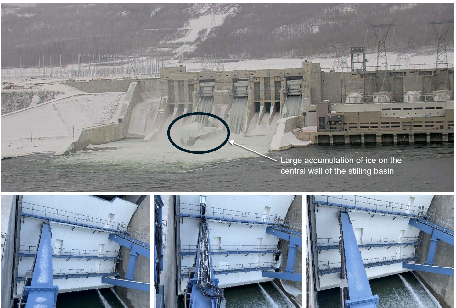
Figure 8 The spillway and spillway operating gates of Site C Dam during winter spill operations. Top: Overview of the spillway showing the very large accumulation of ice on the stilling basin's central wall. Bottom: From left to right, spillway operating gates 3, 2 and 1, showing the absence of accumulated ice on the gates and piers, and demonstrating the effectiveness of the installed heating and operational measures to remove ice.
