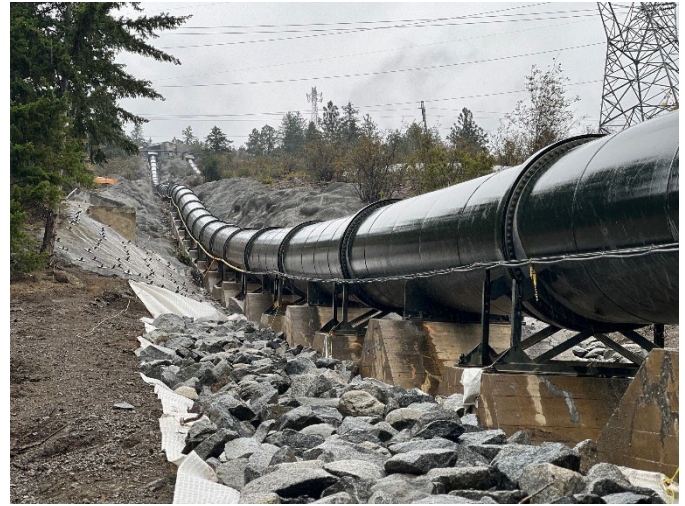
Figure 10 Completed slope improvements and foundation refurbishment on one of the four penstocks at Bridge River 1 Generating Station.
