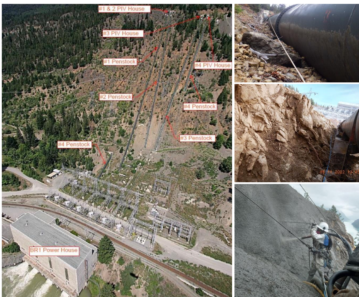
Figure 6 Refurbishment of the Bridge River 1 penstocks. Left: aerial view of the penstocks. Top right: accumulated debris prior to removal. Middle right: penstock trench after debris removal. Bottom right: shotcrete stabilization of penstock trench wall.
