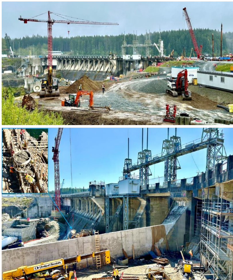
Figure 7 Top: View of the North Earthfill Dam at John Hart, with the upstream berm densification work taking place on the far right and, in the foreground, preparations for the placement for the downstream berm. Bottom: the completed left training wall and concrete placement for the right training wall (inset).
