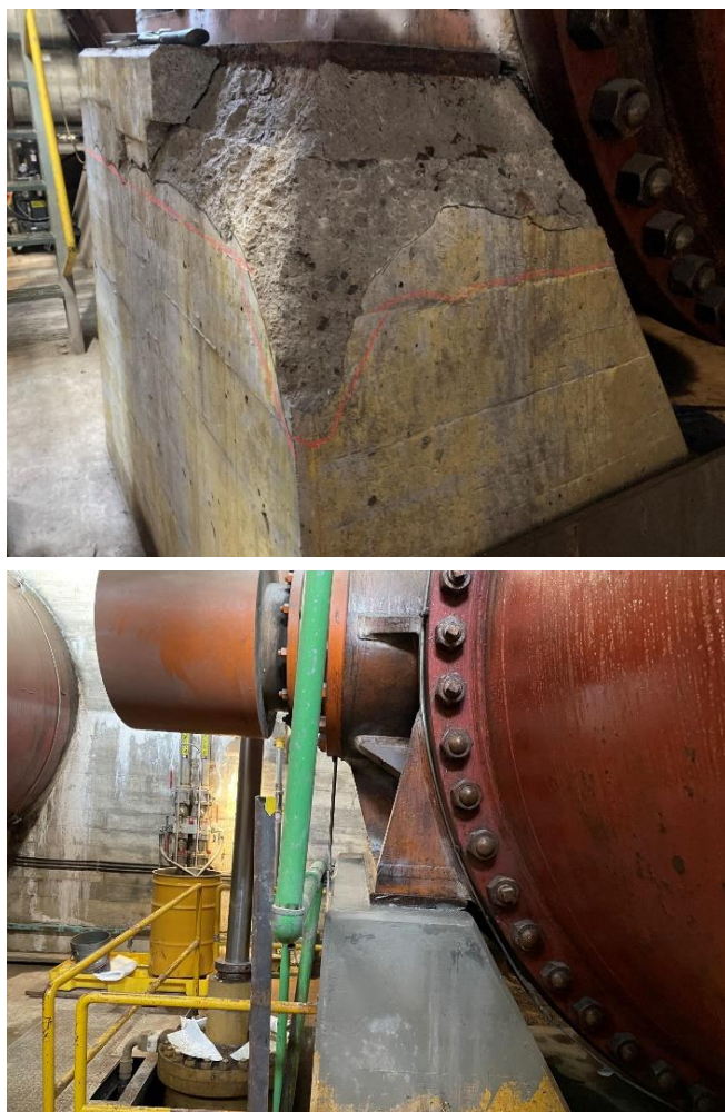
Figure 4 Top: deteriorated concrete pedestal at Bridge River 2 Generating Station. Bottom: concrete pedestal after completed repairs.
