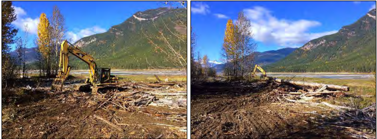
Figure 4-2: Removing wood debris and sorting large logs at the Bush Causeway South site, September 28, 2015.
