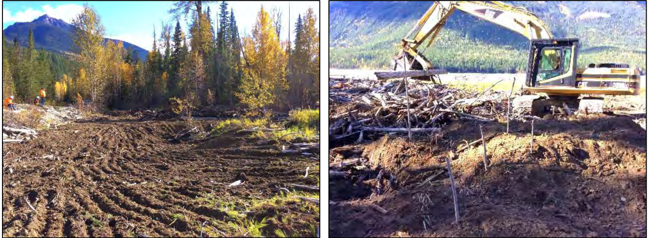
Figure 4-6: Land following de-compaction and furrowing to promote the re-establishment of vegetation at the Bush Arm Causeway South location (left) and live stakes planted in one of the mounds (right).
