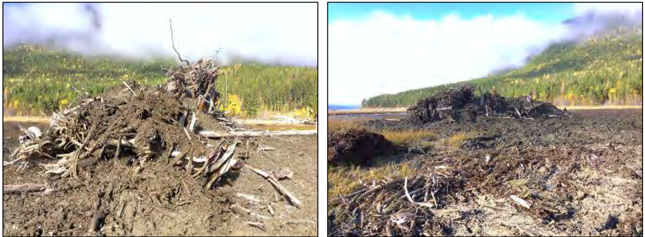
Figure 4-13: Covering the mound with smaller logs and substrate excavated from the site.
