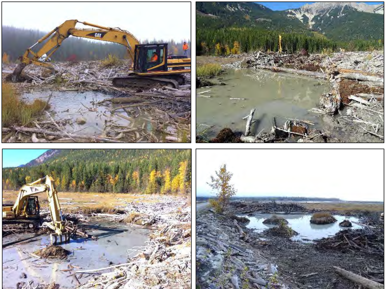
Figure 4-15: Before and after photos of pond clearing and cleanup at the Bush Arm Causeway north location. Note the positioning of a large sill log in the top right. The bottom panels are of the same pond, but from different perspectives to show the wood accumulation (bottom left) and cleaned pond (bottom right) with the retention of peat islands
