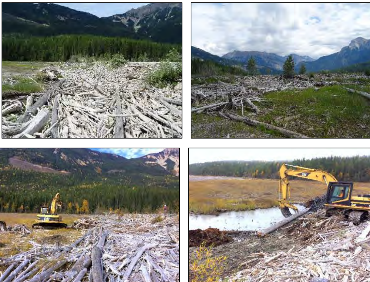
Figure 4-10: Examples of vegetation cover and wood debris distribution at the Bush Arm Causeway North site prior to construction in summer 2015 (top panel) and during construction in the fall (bottom panel). Summer photos dated July 15, 2015; fall photos dated Sept. 30, 2015.
