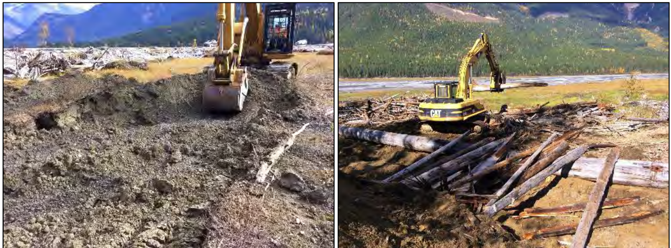
Figure 4-3: Excavating the 'nest' for the sill logs and fill (left) and placing the sill logs and perpendicular base logs at the mound at Bush Arm Causeway South.
