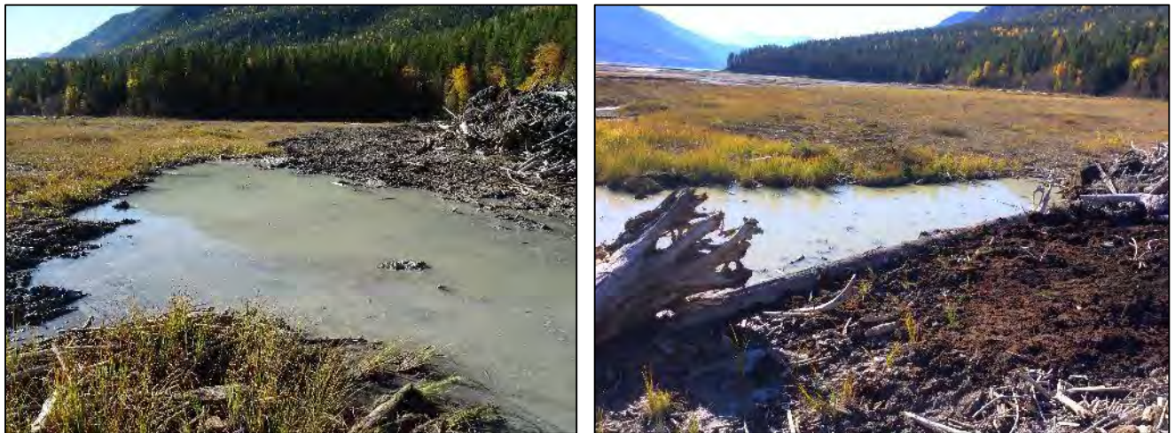
Figure 4-17: Completed physical works at Bush Arm Causeway North showing a cleaned pond (left) and land prepared the re-establishment of vegetation (right, foreground)
