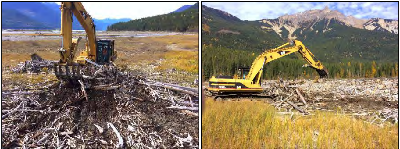
Figure 4-11: Removing wood debris and clearing the ground at the Bush Causeway North Site, September 29, 2015.
