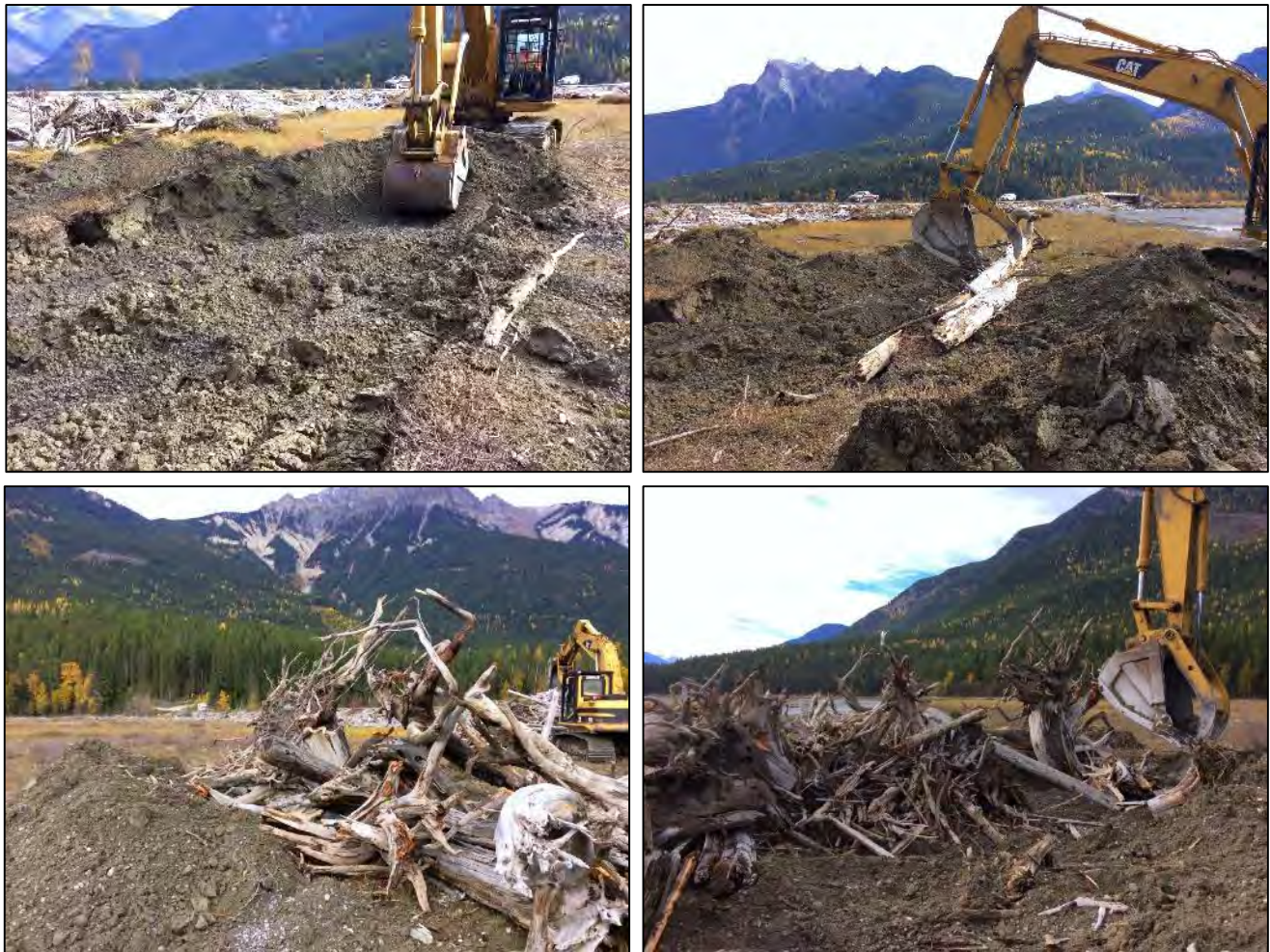
Figure 4-12: Excavating the 'nest' for the sill logs and fill, and placing the sill logs and anchoring the root wads are log logs by back filling the area behind the root wad.
