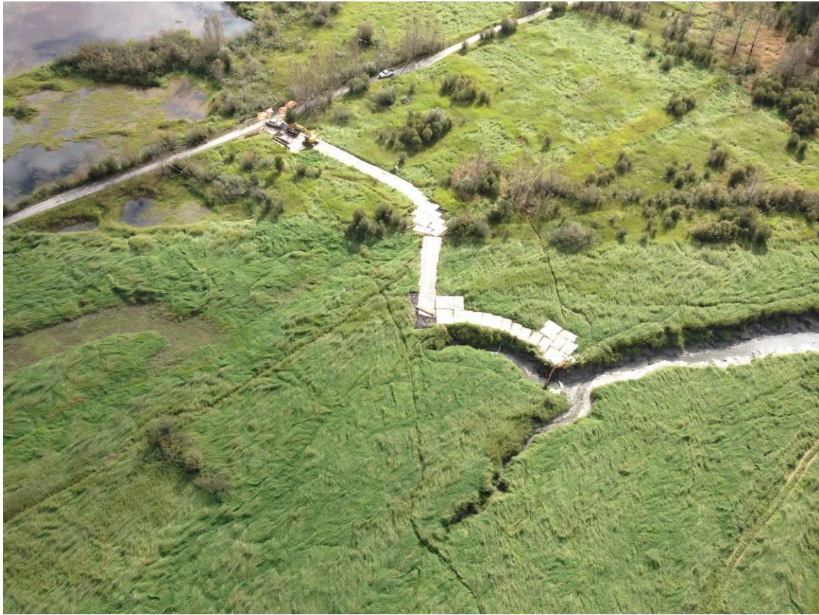
Figure 4-1: Early phase of construction at Wildlife Physical Works site 6A, fall, 2013. The goal of this CLBWORKS-30 project was to prevent an eroding channel from extending towards the Airport Marsh, via the Machete Ponds. The Machete Ponds are seen in the upper left corner
